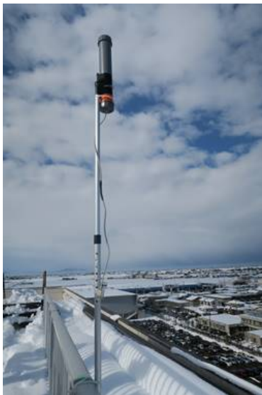
Receiver installed on the roof of the Akiha Ward Office
